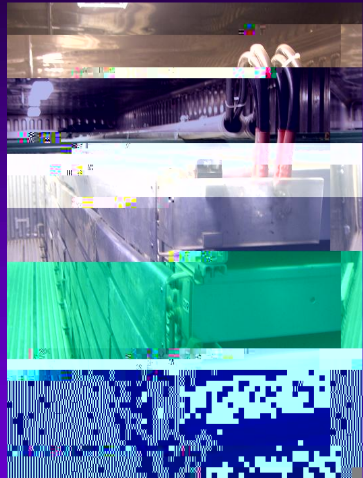
Batteries 3MW Total
