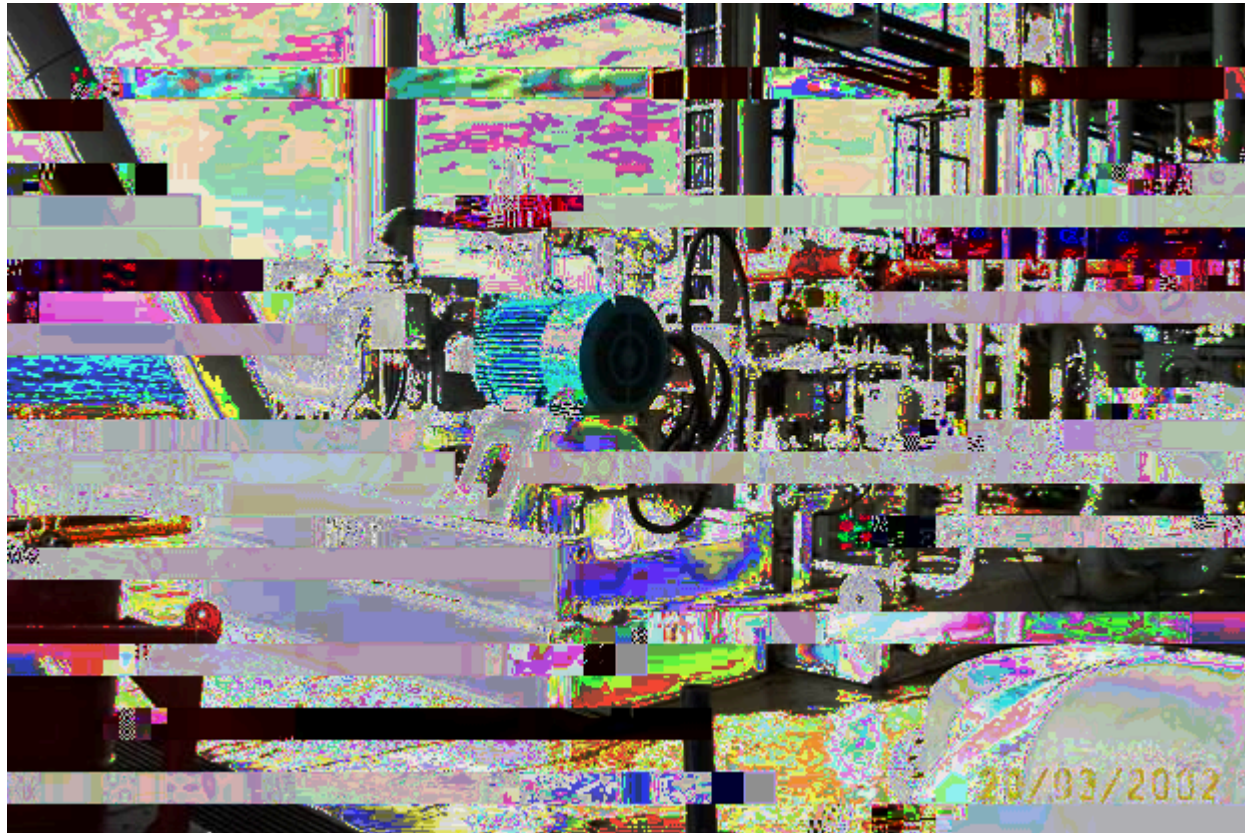
Three-Phase Separating Turbine on Ewing Banks Platform. After Dresser-Rand
